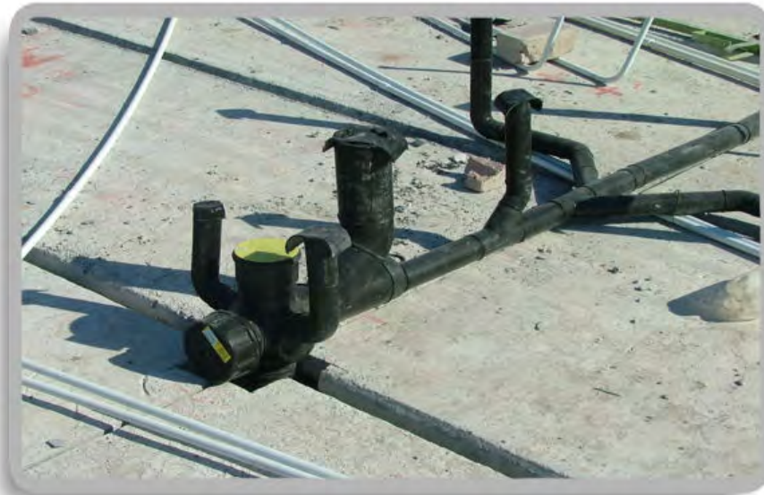
Plumbing and electrical conduits placed prior to screeding. Conduits should be run over the top of the Topfloor slab.
